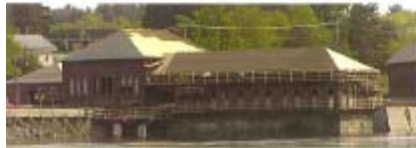
A Bank-financed project will transform the Bangor Waterworks into 25 units of new low-income housing.
